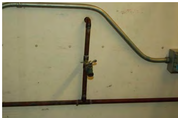
Figure 7. MACC's water pipe and hose bib.
