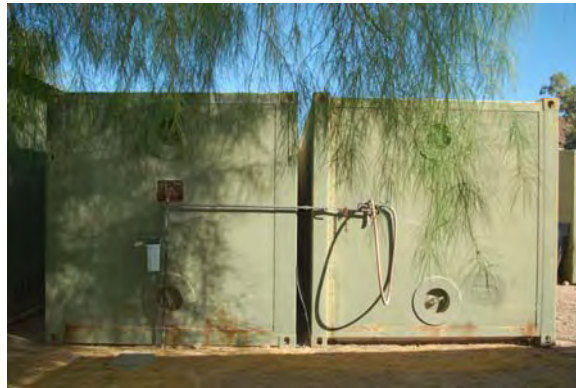
Figure 3. Back view of the MACC shows where water is plumbed into both buildings via pipe.
