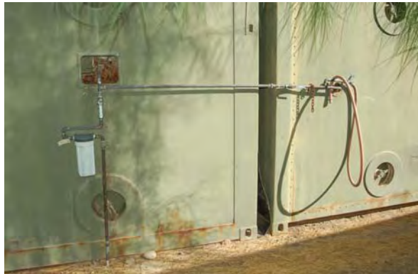
Figure 6. Water supply and filter into MACC
