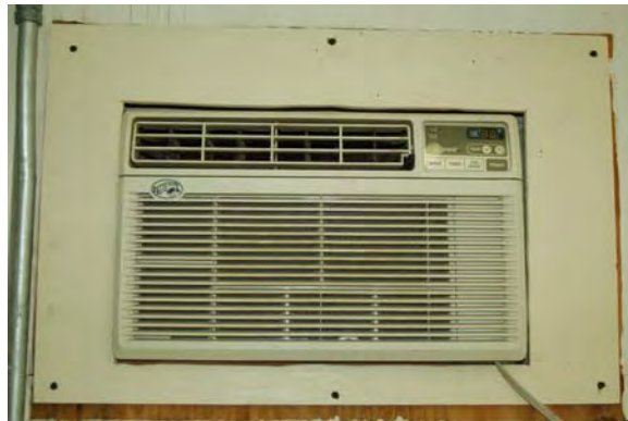
Figure 9. A standard household window A/C unit was installed in the wall of each container.
