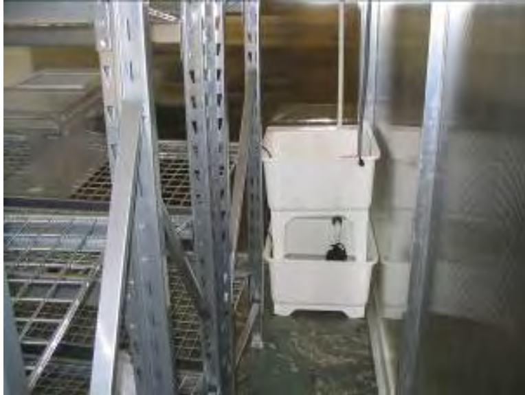
Figure 7. IAR wastewater collection tub with sump pump below.
