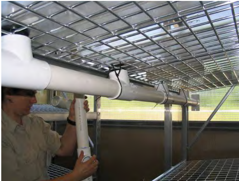
Figure 6. The over-sized drain system under each shelf being installed in the IAR.
